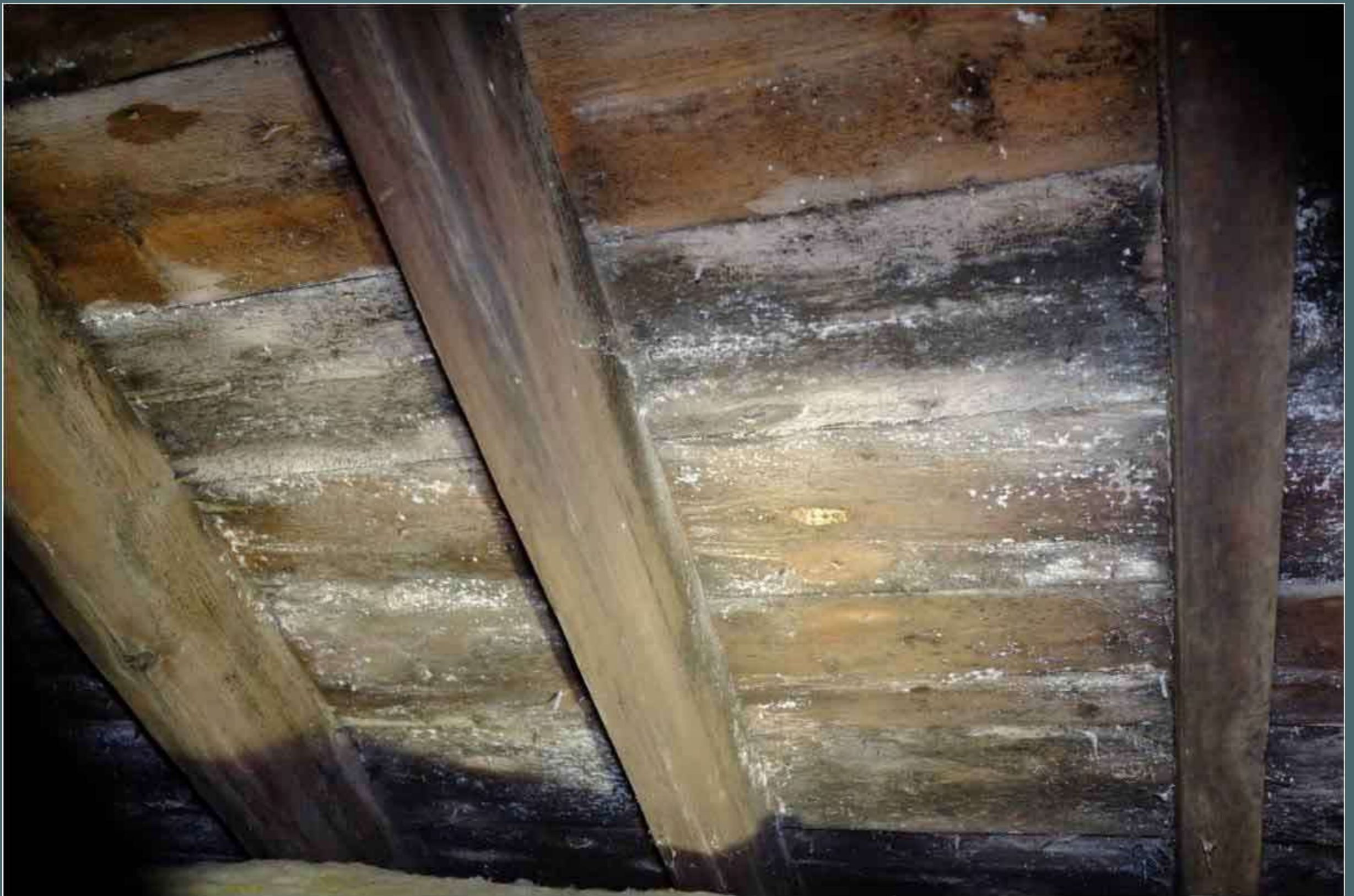
Effect of condensation on roof timbers
