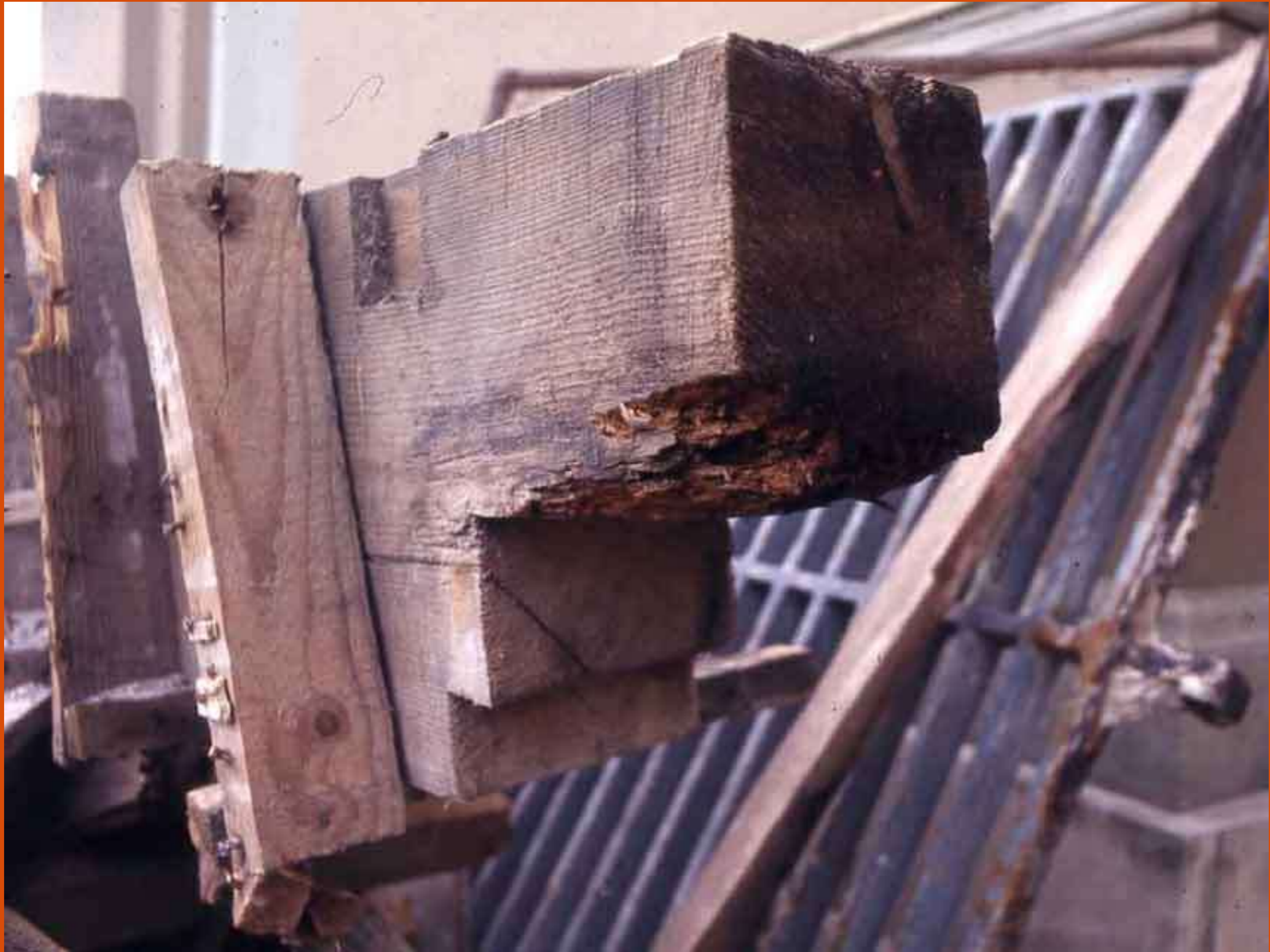
Rot in Bressumer beam ends
