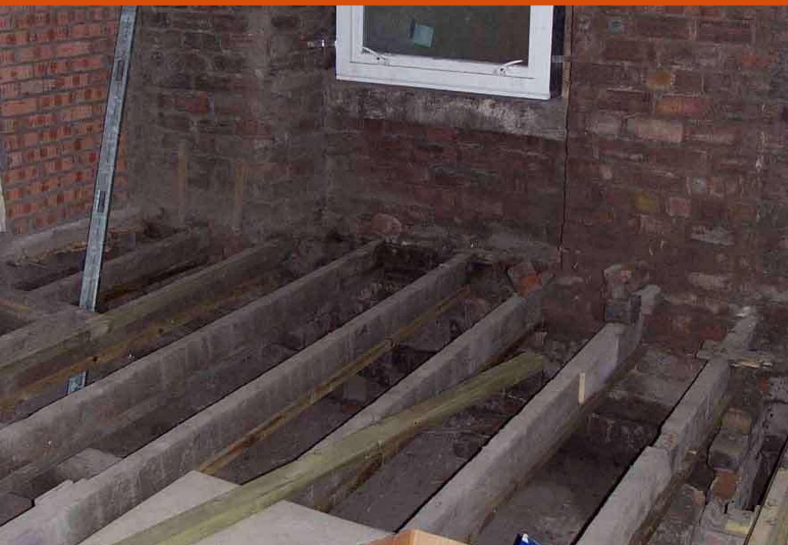
Ground floor joists vulnerable to rising damp
