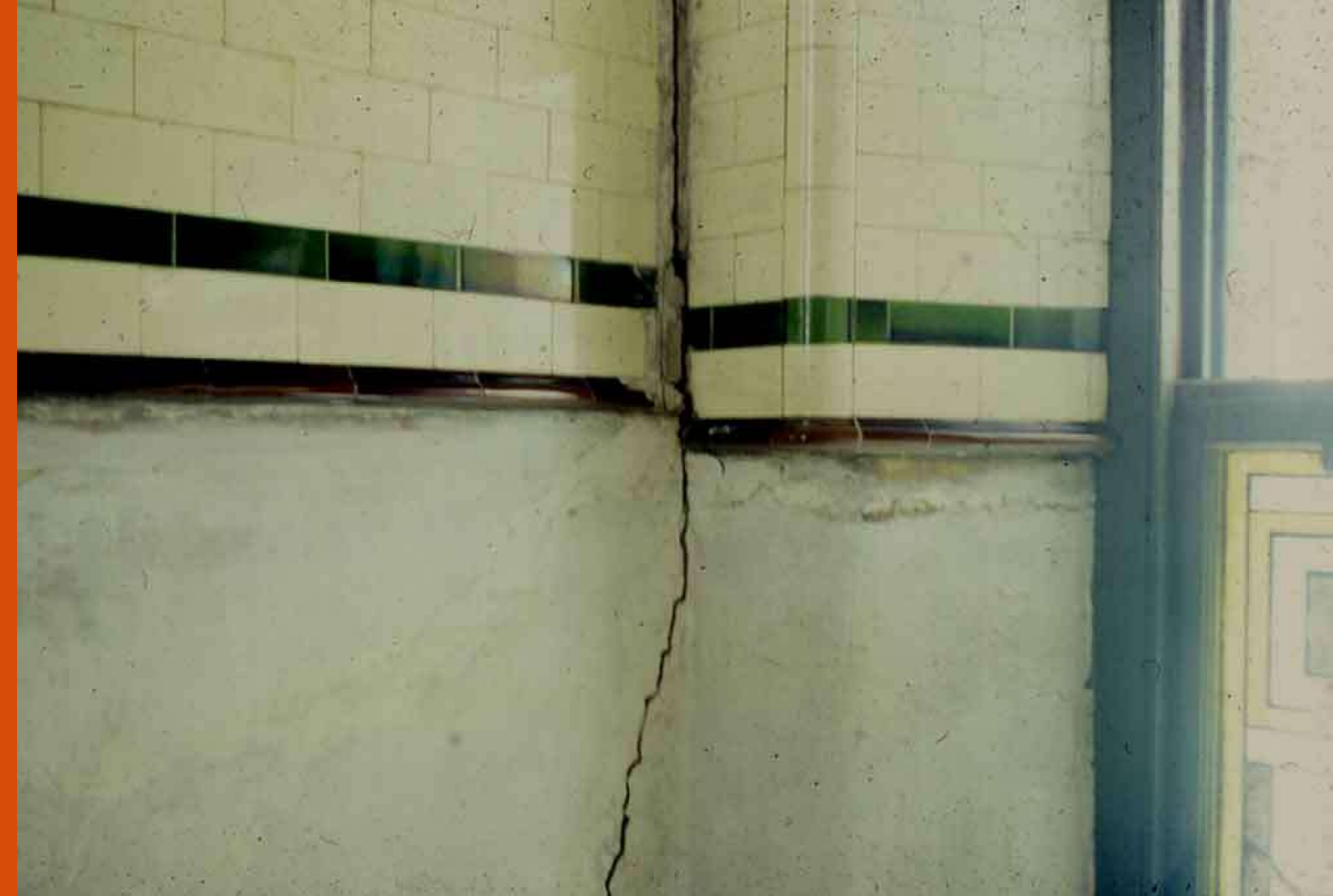
Separation cracks in closes – heavy outer walls sink more than lighter inner walls
