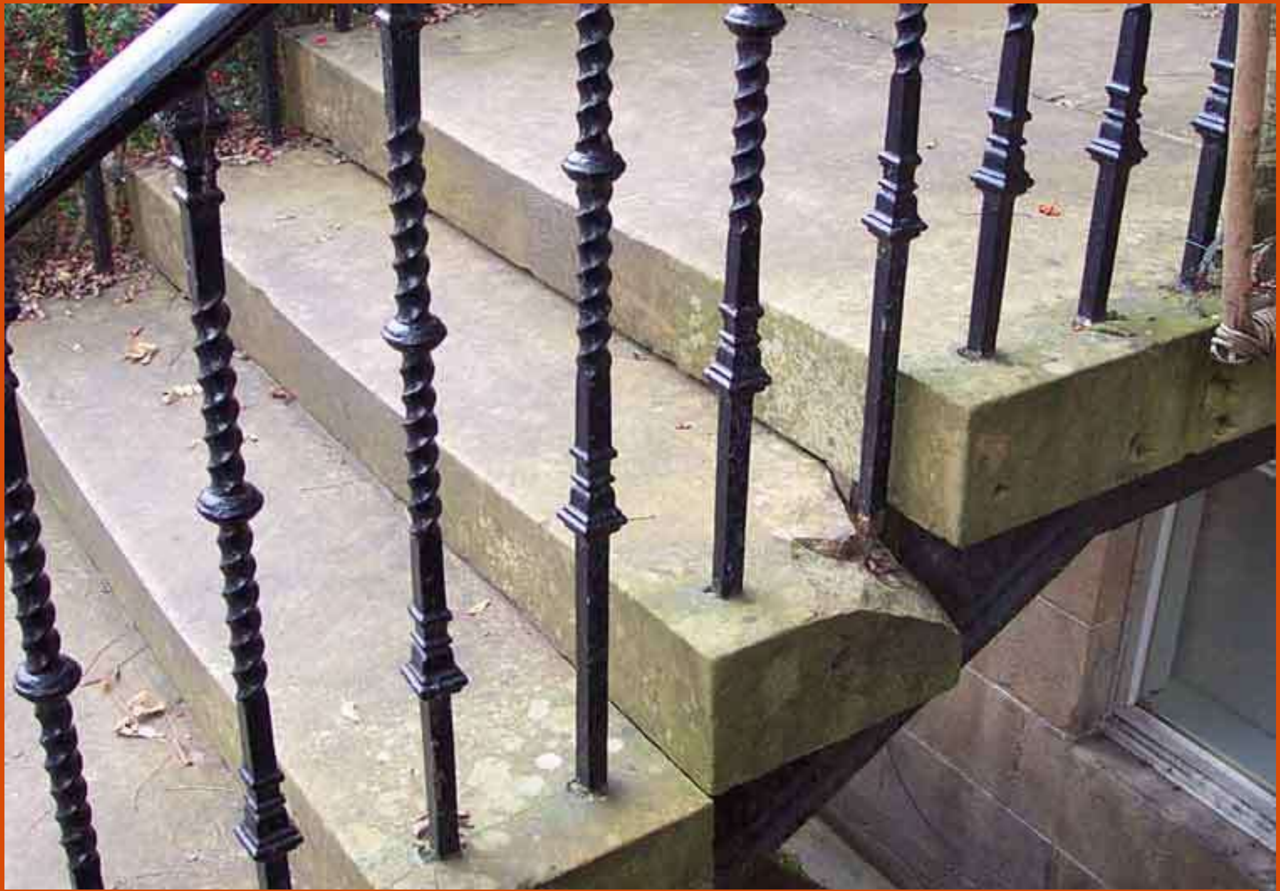
Ironwork – rusting can split stone
