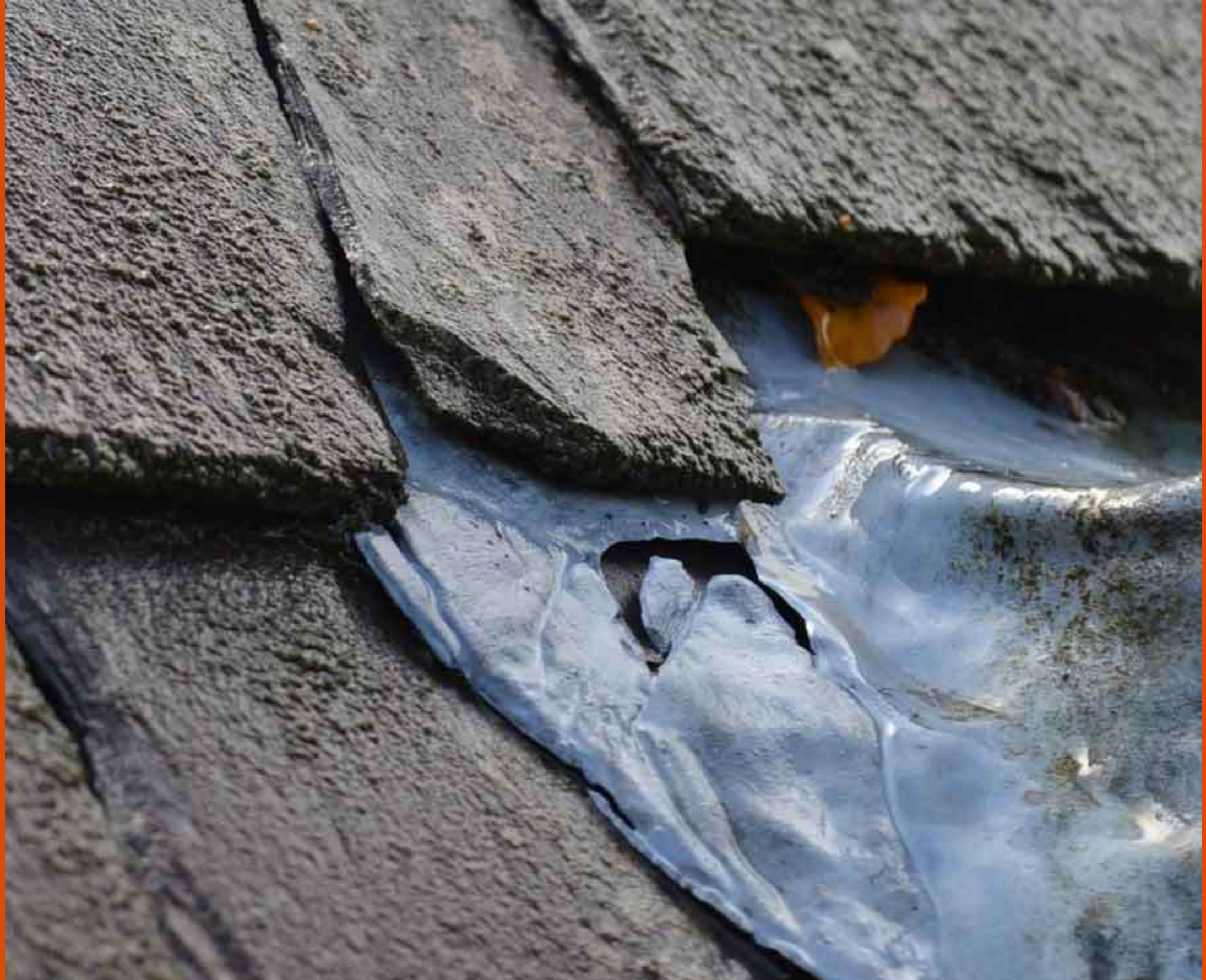
Flashings - Lead may be too thin or badly formed
